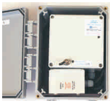
Receiver with logger in protective housing
