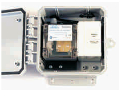
Transmitter in protective housing
